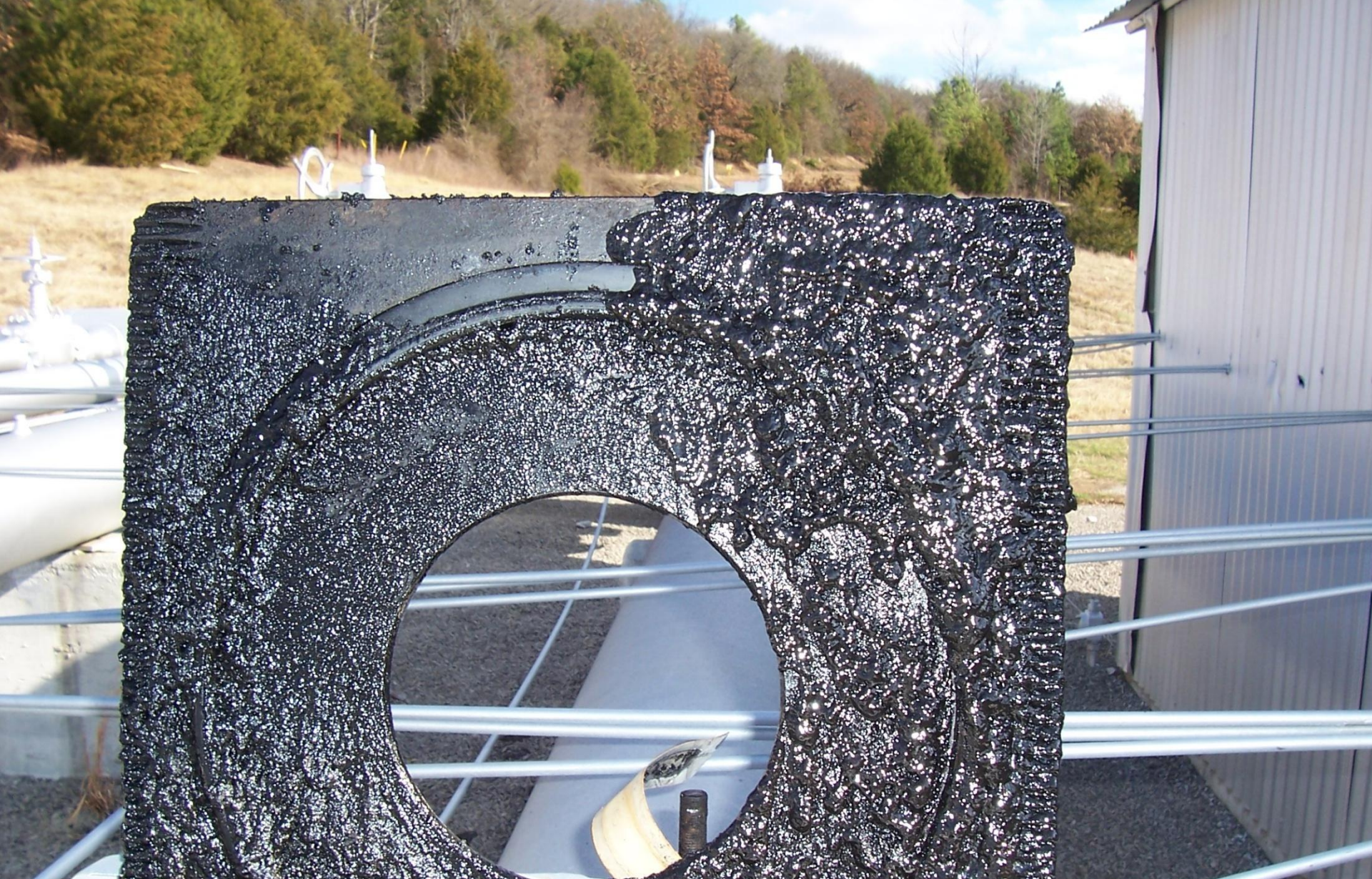
Photograph of Orifice Plate showing example of “Elevated” debris accumulation
